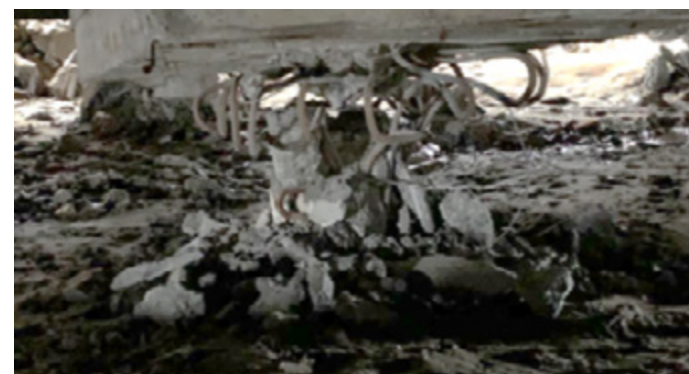
Fig. Failure of some of the reinforced concrete piles which supported the tank.
